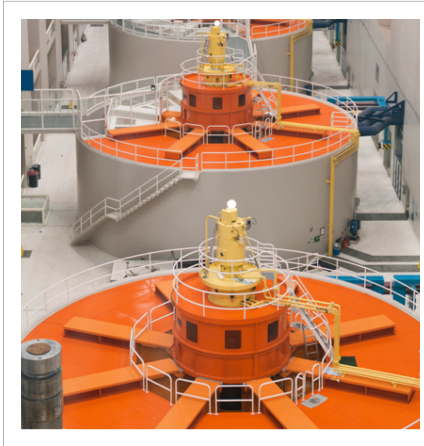
Maintaining high reliability of equipment requires monitoring performance and condition.
