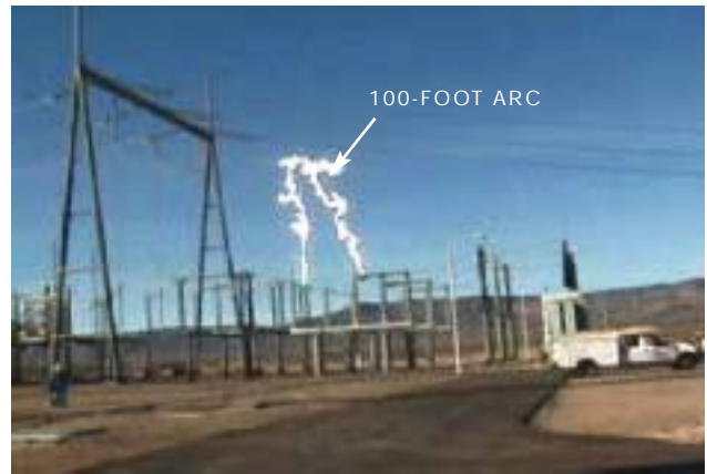
Figure 1 A switch failure at the Eldorado substation in Boulder City, NV, sent this 100-foot long, 500-kV arc into the air (courtesy Stoneridge Engineering, www.teslamania.com ).
