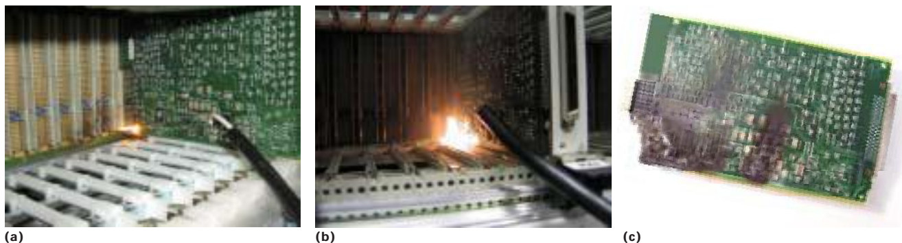
Figure 4 Without proper current limiting, a shorted capacitor in the 5V-dc circuit of a pc-board assembly can start a fire within seconds (a). After 30 sec, the fire has caused considerable damage (b), destroying the pc board and connector (c).
